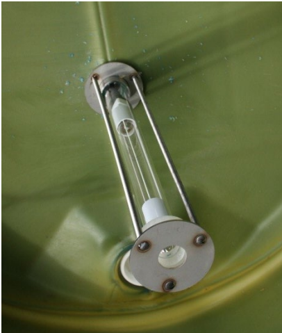
UV unit seen from below – inside tank
